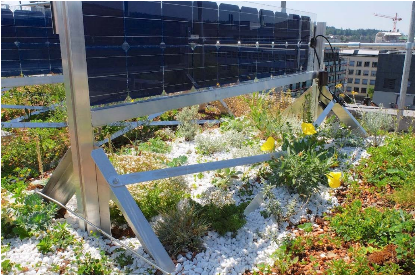
Figure 18: Installation test de la ZHAW, source: Solarspar
